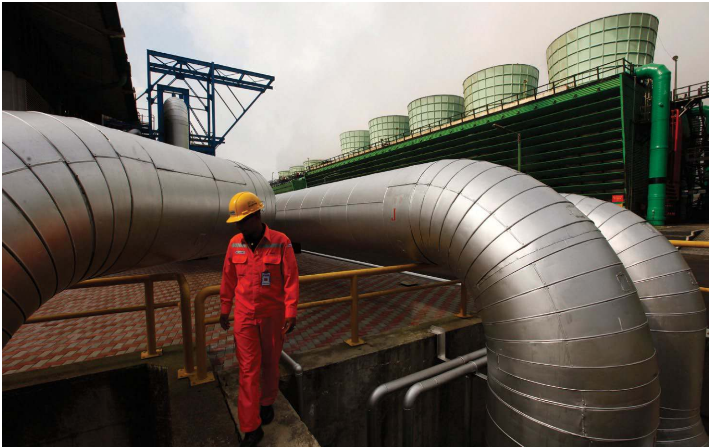
An employee of PT Indonesia Power walks near a thermal pipe at Kamojang geothermal power plant near Garut. REUTERS/Beawiharta Beawiharta
